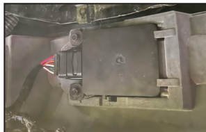
Figure 1: The module is installed facing the wrong direction.
